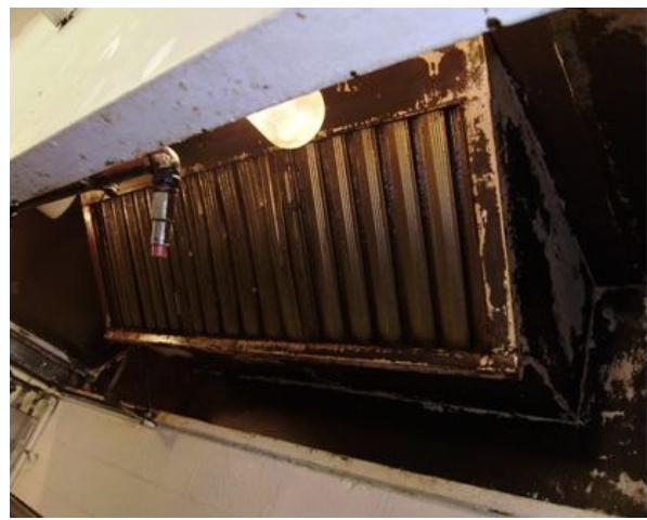
Excessive Grease Buildup
