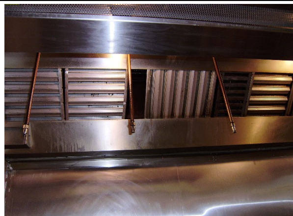
Filters Installed Incorrectly
